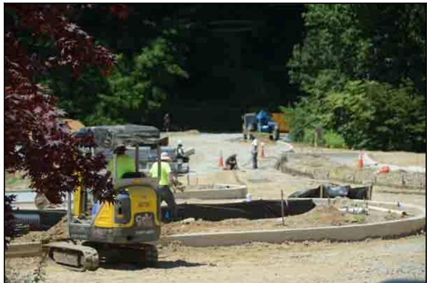
Figure 17.25 – Entrance and Parking Lot Expansion Construction – In 2015, the entrance (Phase I) and the parking lot expansion (Phase II) were combined and completed as one construction project. Source: author – [file:\BSG-065.pdf]
