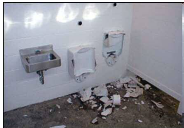
Figure 15.16 – Broken toilet – Caption: Malicious vandalism can be extremely destructive and costly as demonstrated in the destruction of this restroom facility. – Source: Friends of the Rappahannock – [file:\MaliciousVandalism01 .jpg]
