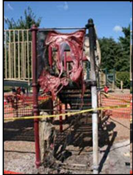
Figure 15.13 – Vindictive Vandalism – Caption: This playground equipment was destroyed by a discontent employee. Baltimore, Maryland. – Source: Internet – [file:\BurntPlaygroundEquip.jpg]
