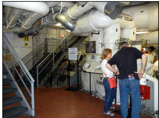
Figure 14.40 – USS Midway Stairway – Caption: Converting historic facilities that are designed for a different purpose can be expensive and difficult to install. The stairway in the back of one of the engine rooms in the USS Midway was added to provide access by the general public. USS Midway, San Diego, California. – Source: author [file:\fig1336-DSCN0557.jpg]
