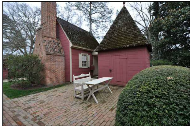
Figure 14.3 – Outbuildings – Caption: Traditionally, outbuildings are not constructed with longevity in mind. Examination of these two outbuilding next to the Wyrth house reveals that they are not built on substantial foundations and that the wood shingles are moss covered and will soon need replacement. – Source: Author [file:\fig1303-WB036.jpg]
