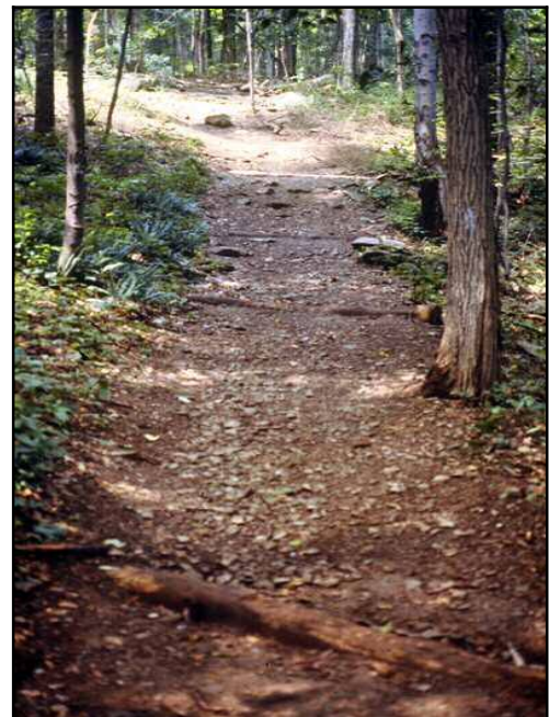
Figure 13.32: Multiple waterbars – A series of waterbars placed on the trail to divert water off the trail before it can gain sufficient power to erode the trail. Gambrill State Park, Maryland. – Source: Author – [file:\waterbars.-multi.jpg]
