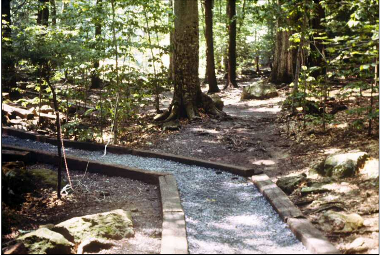
Figure 13.26: The Old Trail – The trail is well defined with the limestone surfacing and the railroad tie stringers. The old trail to Cunningham Falls is clearly visible. A fence or naturalization with plants would help deter use of the old trail and short cut. Thurmont, Maryland. Source: Author – [file:\DSC_0136.JPG]
