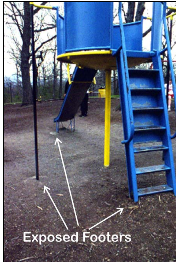
Figure 3.19: Trip Hazards – The exposed footer pose a trip hazard. Twelve inches of mulch would solve the problem. Source: author [file: \PL_Footers.cdr]
