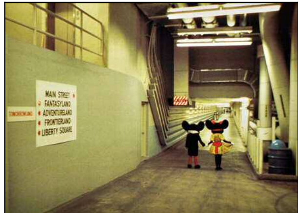
Figure 1.19: Utility Corridors – The “utilidors” or tunnels and other facilities on the first floor beneath main street provide access to the set by actors and support personnel servicing the Magic Kingdom. Disney World, Orlando, Florida. Source: Disney (1986) – [file:\fig0114-Tunnels02.JPG]
